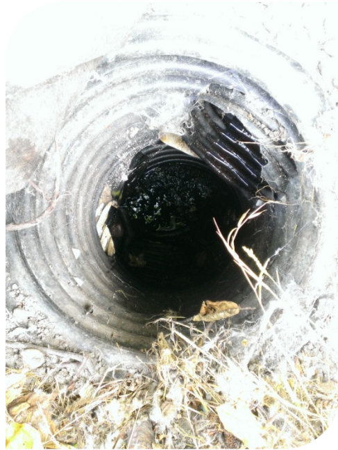
Photo 9— Catch basin collecting roof, driveway, and collection basin runoff.
