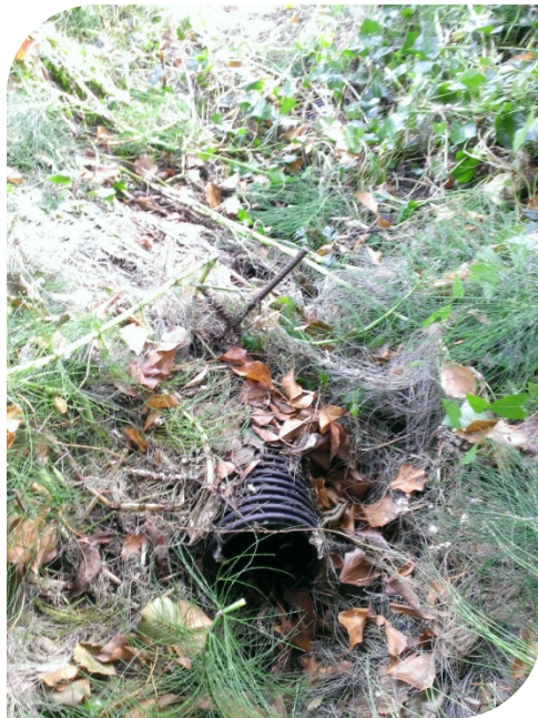
Photo 4— Inlet of runoff collection basin. Note lack of channel.
